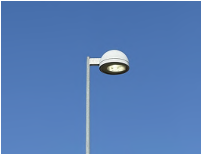
Concord exterior lighting fixture
